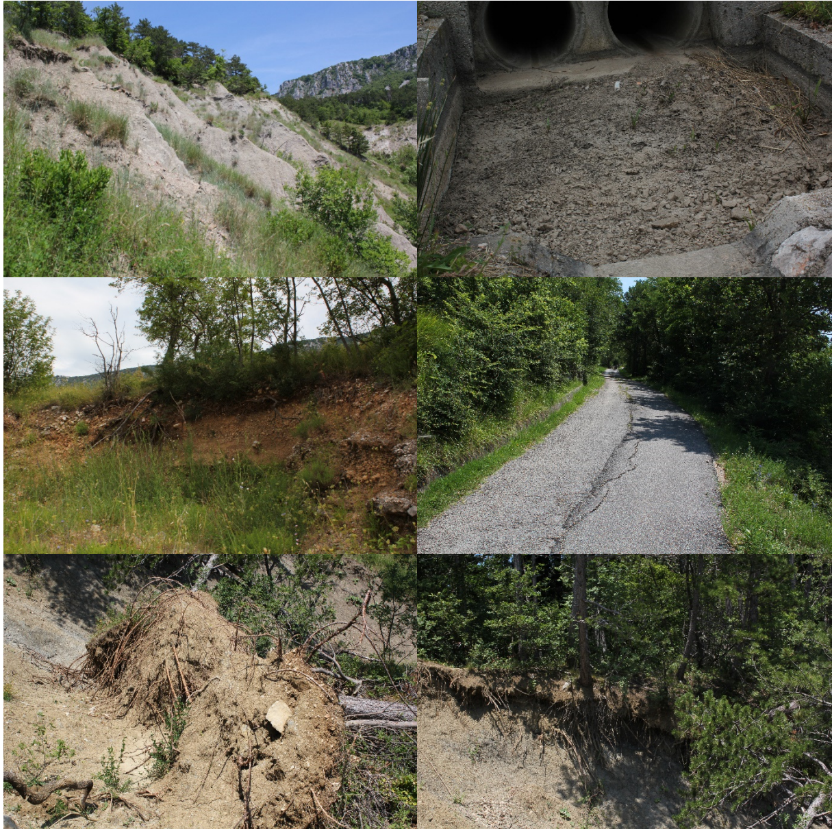
Figure 49: Visual signs of erosion processes captured in field survey in June 2016 (pictures taken by author in July, 2016)
