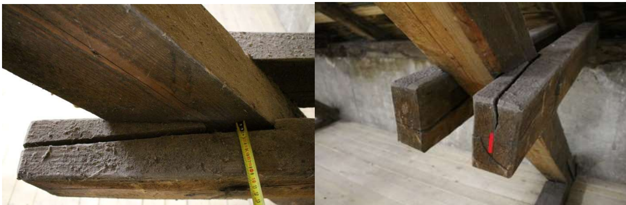
Figure 4.6. Cracks in connection brace-short tie
