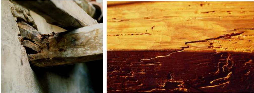
Figure 1.42. left: Decayed beam – result of the fungal attack; right: Cracked beam – indicates a brittle fracture (bending failure) due to the overload [57]
