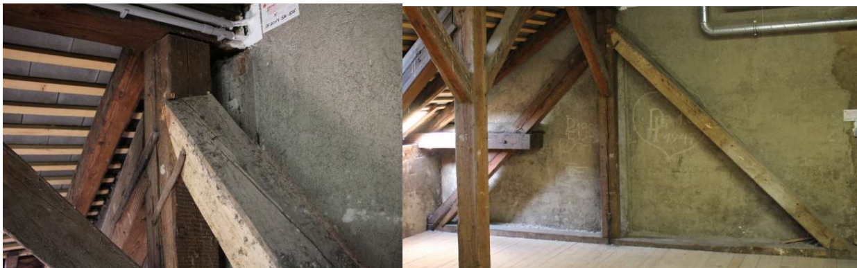
Figure 4.1. left: Connection Brace-Post (Photo:6500); right: Brace on axis 14 (Photo:6644)
