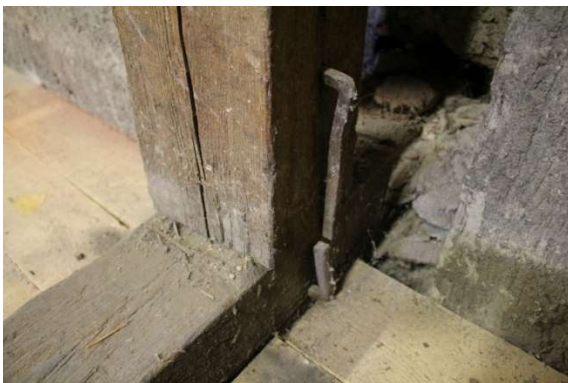
Figure 4.8. Failure of the iron cramp on axis 11 (north post)
