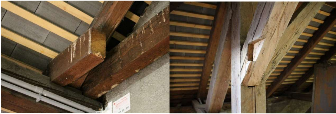
Figure 4.2. left: Cut Collar beam (Photo 6525); right: Damaged Knee brace (Photo: 6624)
