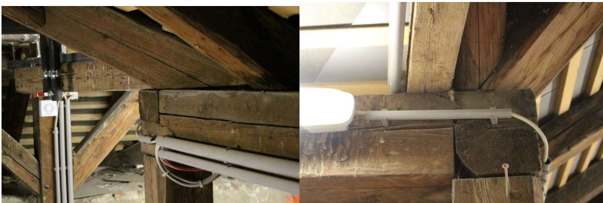
Figure 2.24. left: Half lapped connection with a notch on the upper edge; right: Half lapped connection with a notch on the bottom edge
