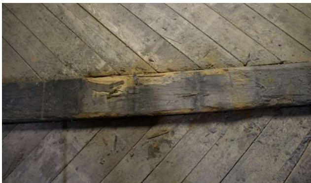
Figure 4.5. Damage to the tie beam due to the House longhorn beetle
