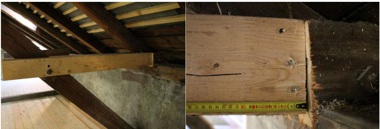
Figure 4.3. left: Changed short tie axis 3 (Photo6604); right: Connection of the new short tie to the old short tie (Photo:6468)
