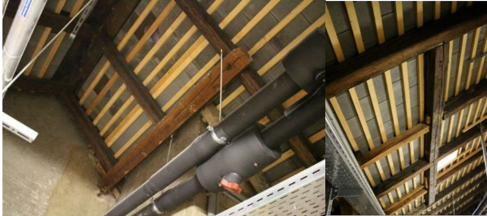
Figure 2.34. left: Transverse beam connected with bolts; right: Transverse beams connected with the tenon and mortise
