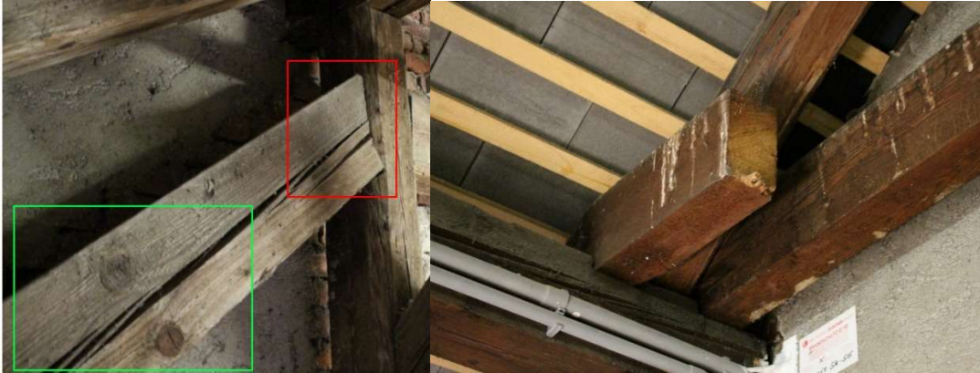
Figure 1.44. left: Cracks in brace at “TU Graz Alte Technik” (green uncritical, red critical) right: Removed collar beam in order to provide room for chimneys “TU Graz Alte Technik”
