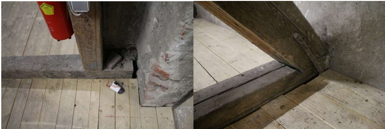
Figure 2.35. left: Visible support of the tie beam to the masonry; right: Support of the tie beam to the masonry hidden in the wall pocket
