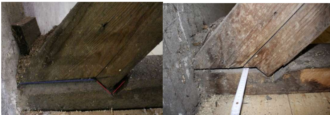
Figure 2.22 left: Rear /heeled notch with marked load transfer planes; right: The gap in notched connection
