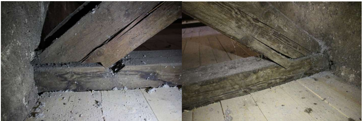
Figure 4.7. left: Partly disconnection of the connection brace-tie beam; right: Cracks due to the load transfer
