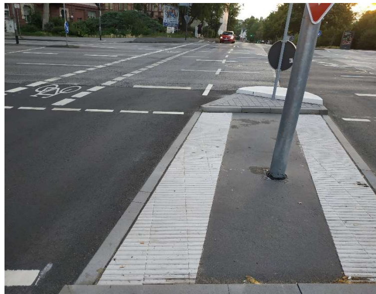
Figure 19: Central pedestrian island
