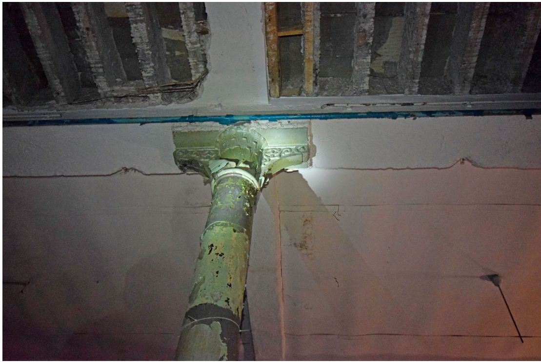
Figure 7. Tobacco Factory T-building, first-floor skeletal structure — detail of capital and pillar (Marko Franković, 2018).
