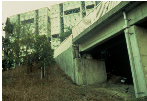
Figure 5. Sliding displacement of a bearing device of bridge superstructure and inclination (damage) of reinforced concrete pier wall, Ashya Seaside Village in Kobe, the 1995 Kobe earthquake;
