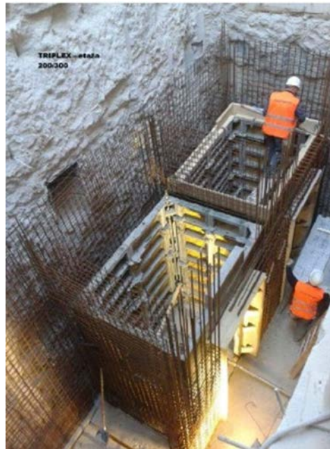
Figure 10. Photo of elevator shaft concreting. D. Sošić: Reconstruction of Hotel President in Dubrovnik in 2013, Master's thesis, University of Rijeka, Faculty of Civil Engineering, Rijeka, 2020.
