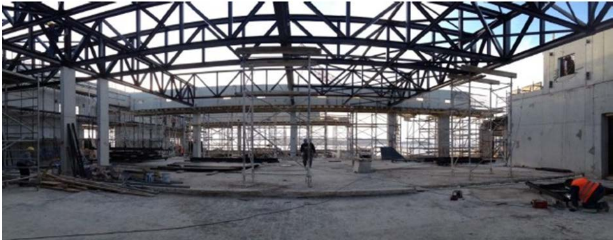
Figure 8. Photo of the lattice roof structure of the hotel reception during the reconstruction in 2013. Studio 92 d.o.o., Labin
