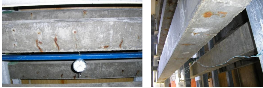
Figure 6. Cracks caused by sustained loading
