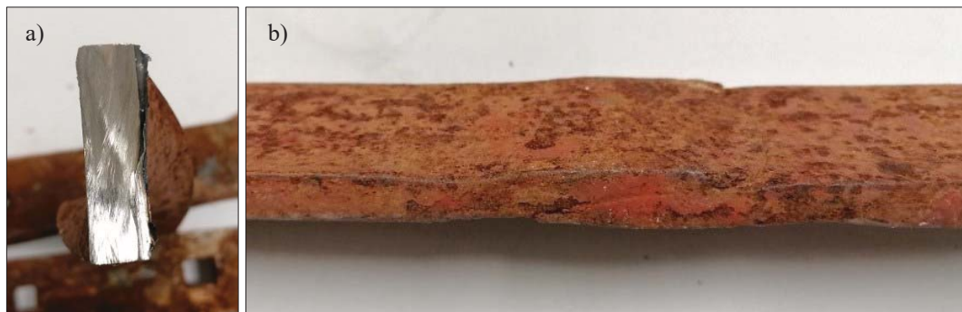
Figure 9. a) Cross section of a diagonal tie; b) Detail of forged connection confirming it is wrought iron.
