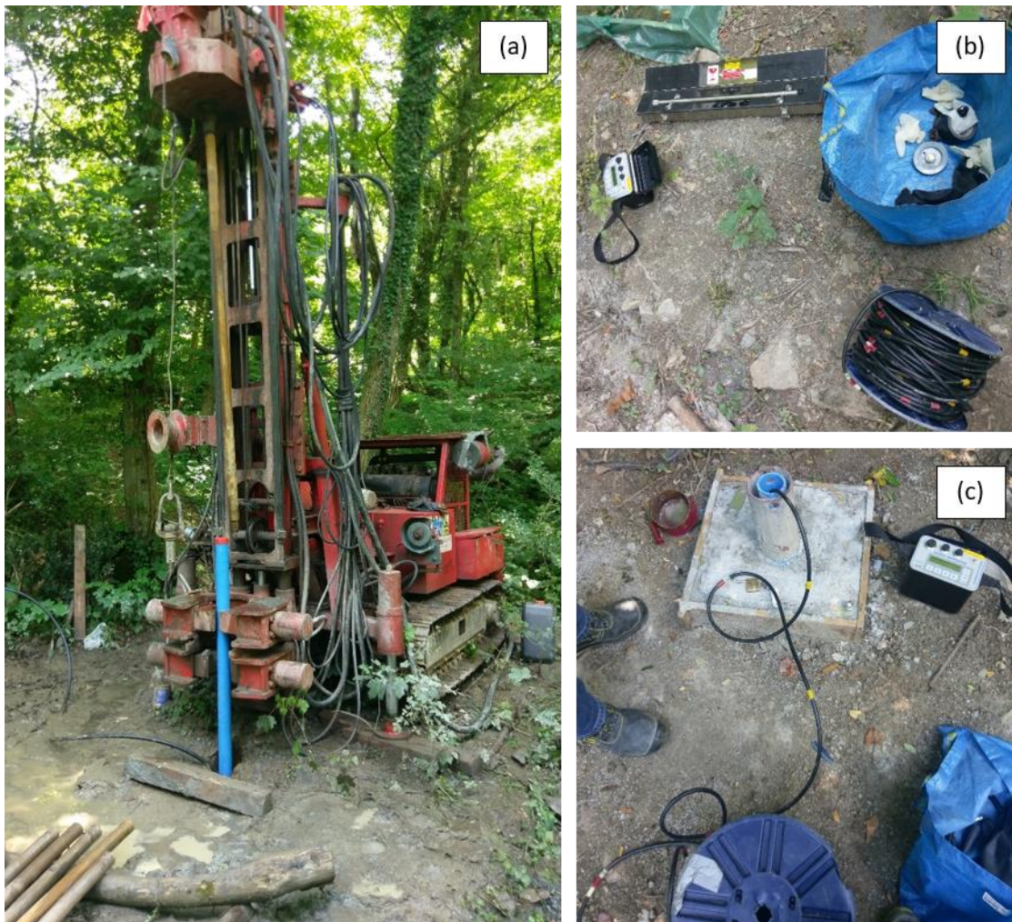
Figure 10: Details of a) inclinometer chasing installation at the B1 location; b) portable inclinometer measuring system Digitilt Classic Inclinometer System (Durham Geo-Enterprises, Inc.); and c) measurements in progress.
