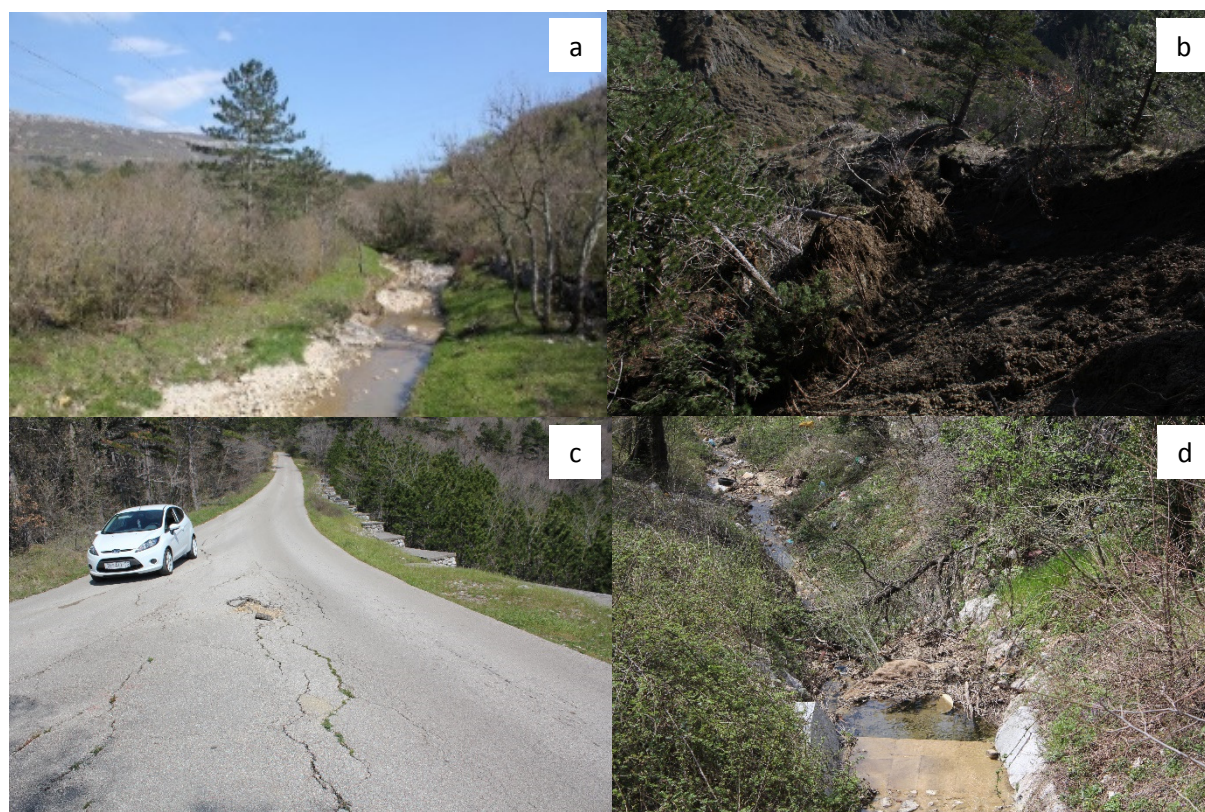
Figure 3: (a) Sediment in tributary Malenica riverbed, (b) Land instability: intensive erosion processes causing local landslides on Slani Potok sub-catchment (c) Road damage due to land instability on border of Slani Potok and Mala Dubračina sub-catchments, (d) Unmaintained river bed of one of the Dubračina tributary's [photographs taken by author]
